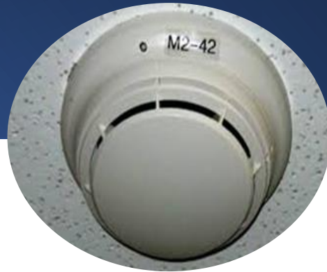
Typical Building Fire Alarm Smoke Detector
