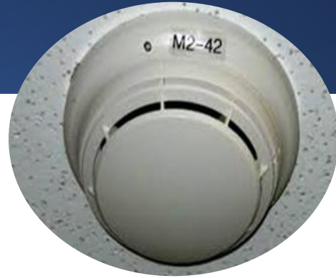
Building Fire Alarm
