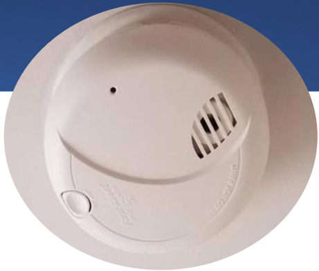
Typical Suite Smoke Detector
